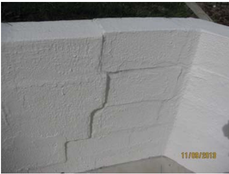
Structural Damage to a Retaining Wall
