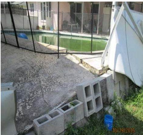
Heaved pool shell and slab
